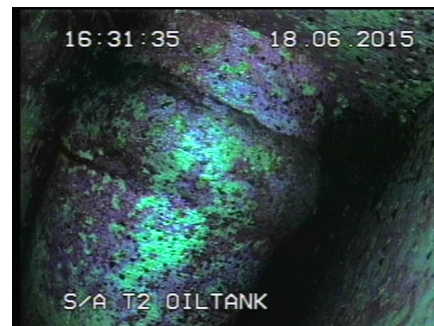
Fig 3d: Extensive corrosion on inner pipe
