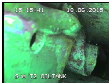
Fig. 3c: Corrosion and debris on baffle plate
